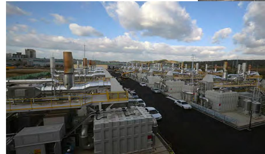
The world's largest operating fuel cell power plant (59 MW), located in Hwaseong, South Korea
